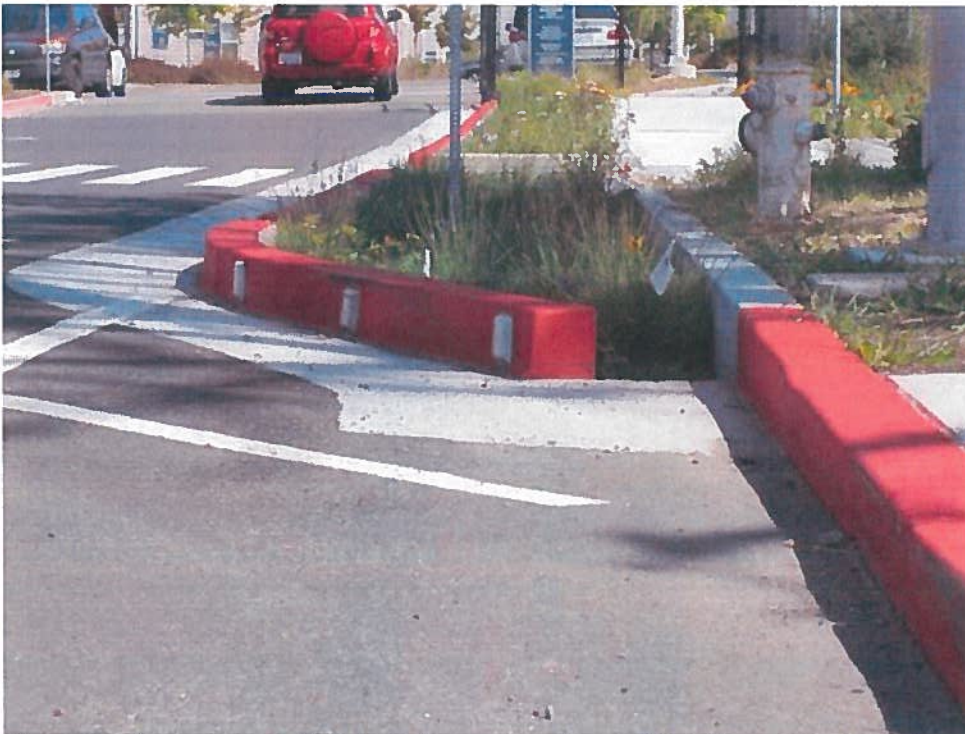
Figure 2: In-line system in Berkeley/Albany where low and high flows enter the system and overflows exit through a drain within the system.
